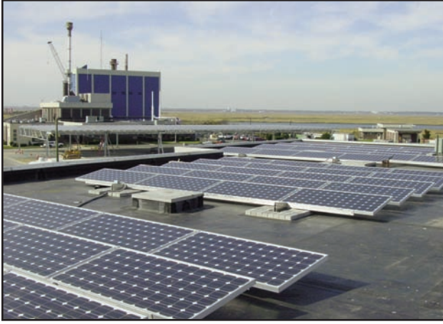
The ACUA has teamed up with World Water & Power/Conti/Alternity to build a 500-kilowatt photovoltaic solar project.
