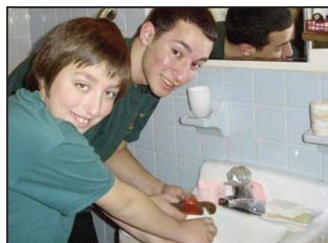
Two Scouts help retrofit a unit in the New York Ave. apartments in Atlantic City.
