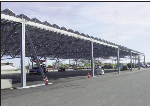
The project consists of two ground mounted arrays, two roof mounts and a canopy array built to cover the parking lot.
