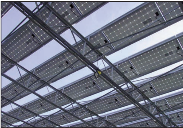
The roof mounted canopy arrays will be mounted on non-roof-penetrating brackets ballasted to withstand hurricane force winds.
