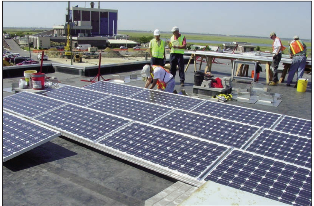
The installation of 2,700 solar panels began September 2005 at the Atlantic County Utilities Authority Wastewater Treatment Facility in Atlantic City, NJ. The 500 kilowatt (DC) system was completed in June 2006.
