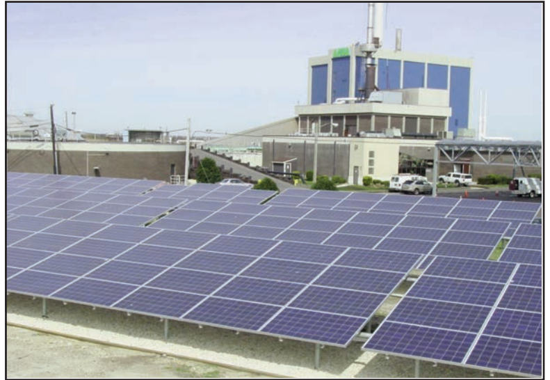
Solar panels are located on the ground, roof tops and as a canopy over the employee parking lot at the ACUA's Wastewater Treatment Facility.
